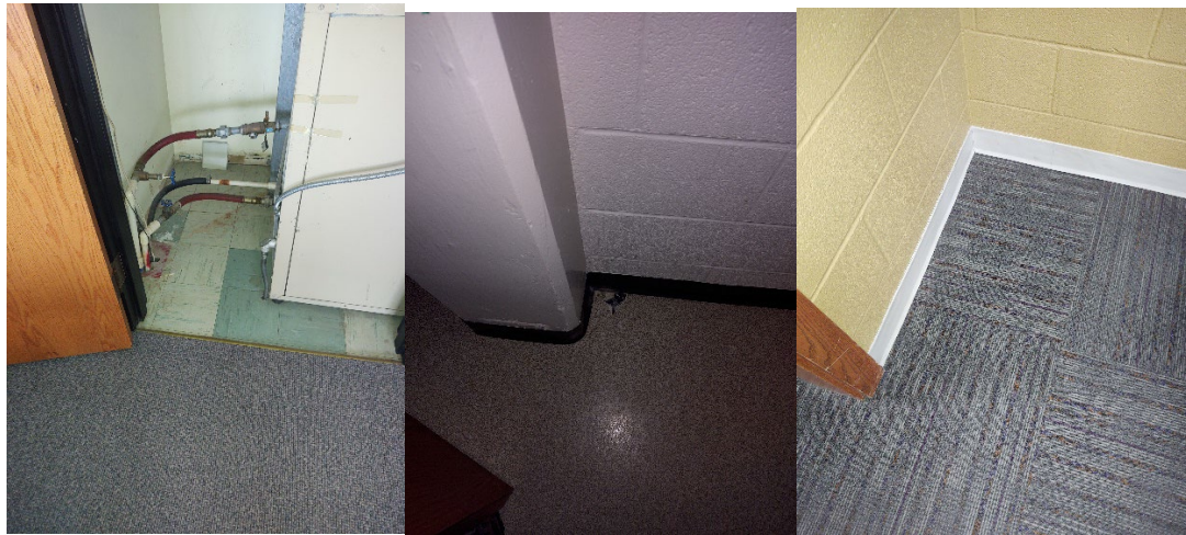
Tile in closets under carpet with black mastic, ACM seamless flooring above 9 inch tile
