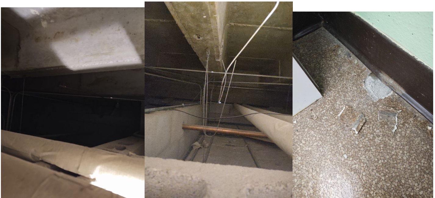
ACM Sheet flooring in Morgue
