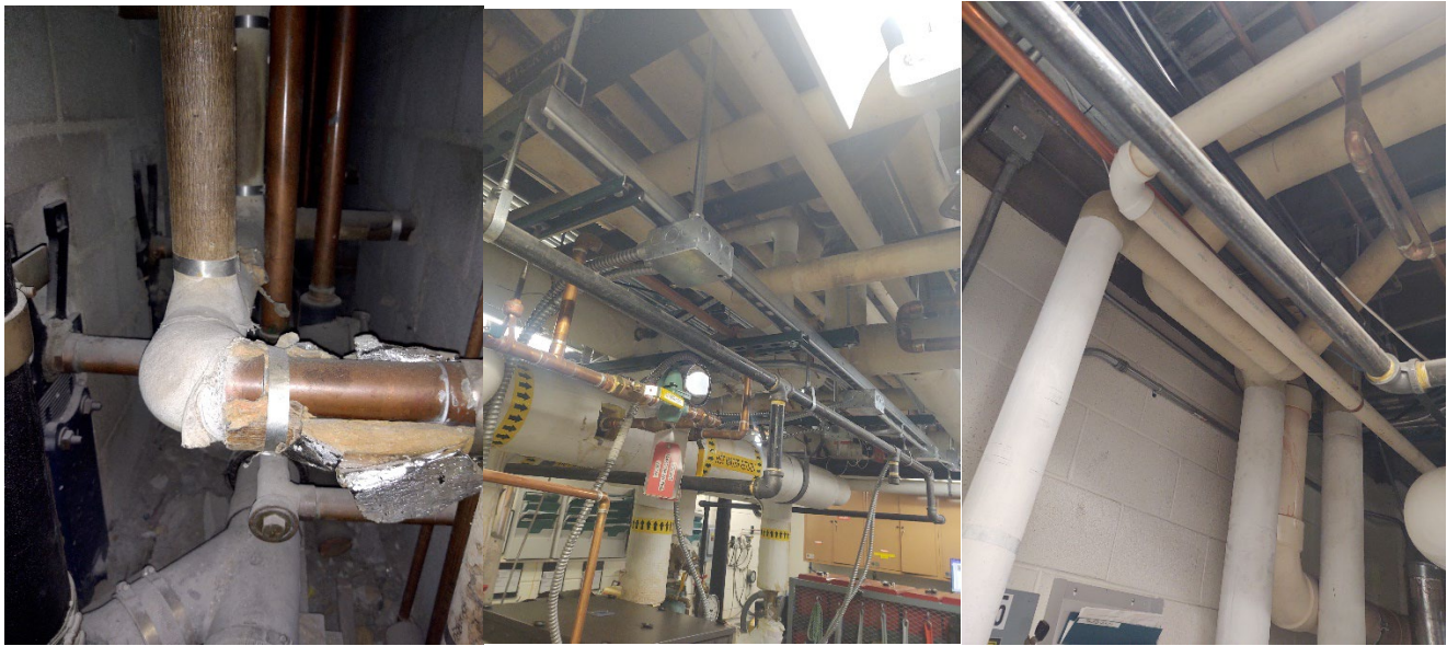
Tsi pipe insulation
