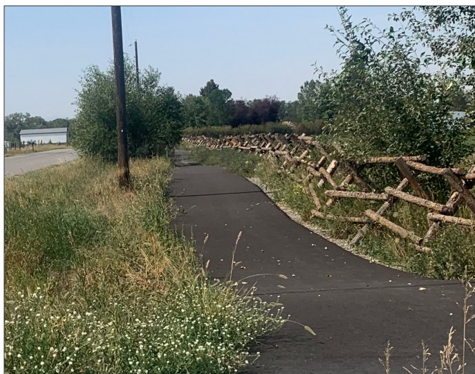
Good initial planning, proper design, and regular maintenance can help extend the life of shared use paths.
